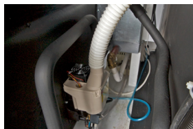
Tubing and cabling
