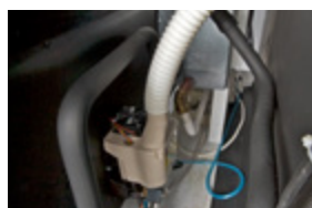
Tubing and cabling
